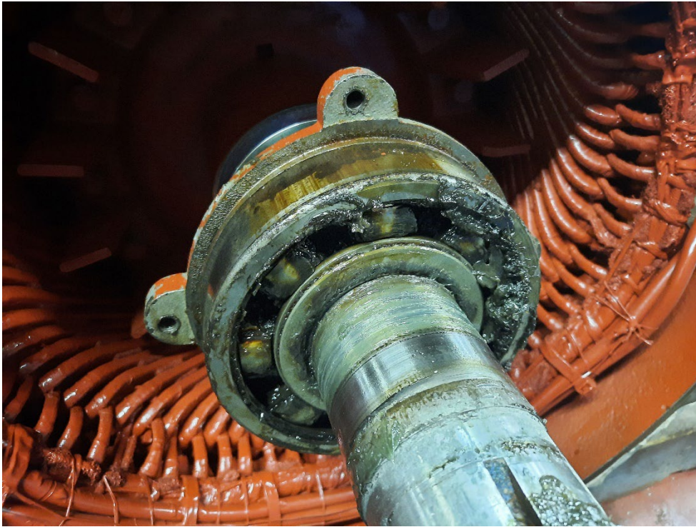
Figure 8: Opposite Drive End bearing grease and fretting on the outer race. Grease is caking and oil separating.
