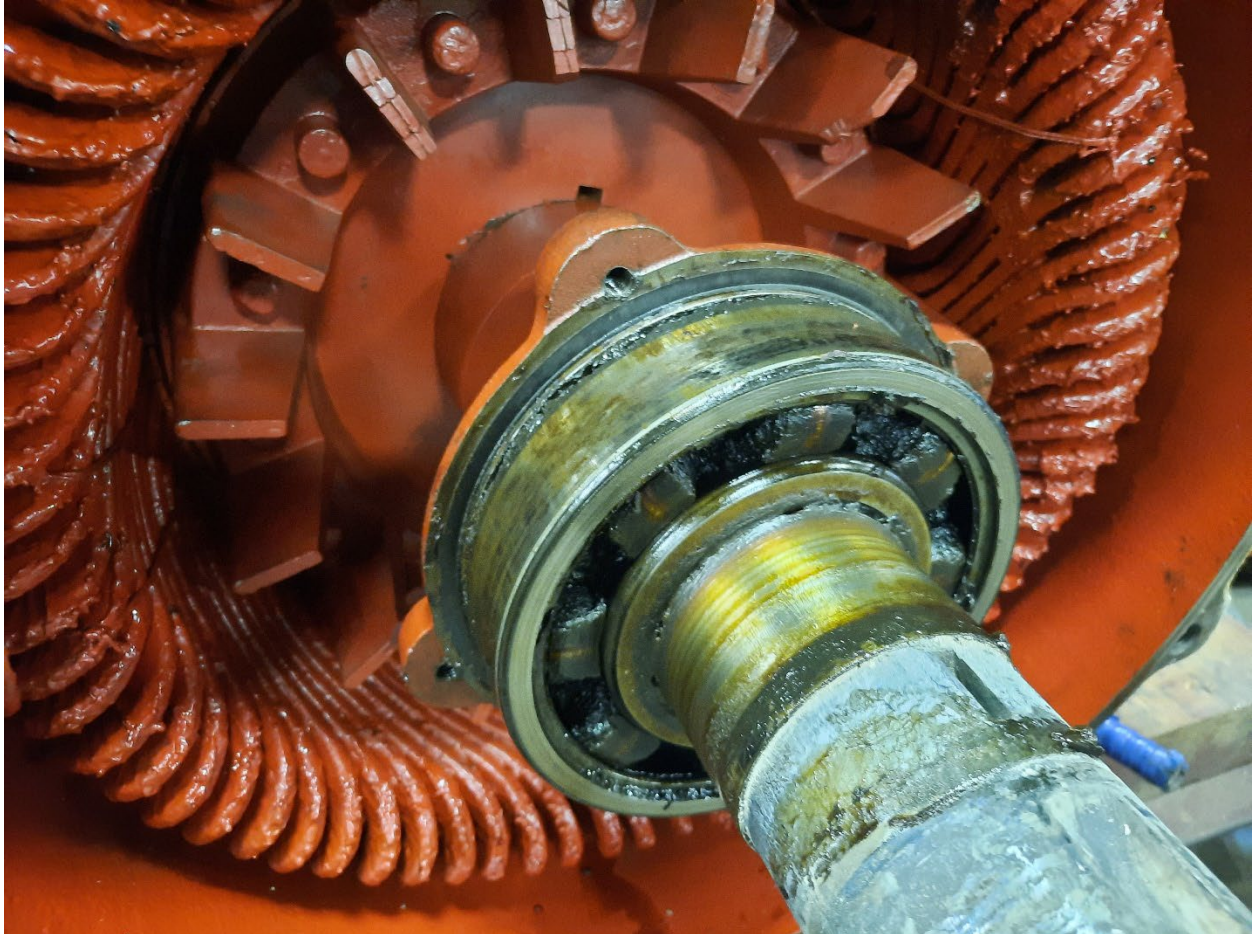
Figure 7: Drive end bearing and rotor once the end shield was removed.
