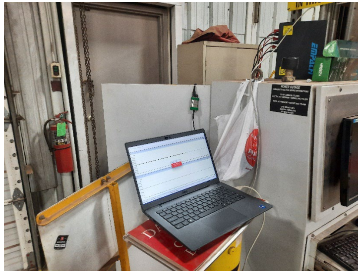
Figure 3: EMPATH data collection upper right and laptop with the EMPOWER hanging over the door of the back of the test panel controls.
