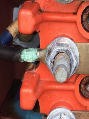
Removed Insulation to find Corrosion
