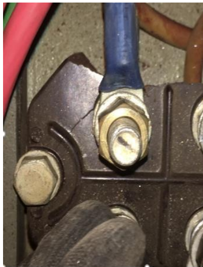
Broken terminal block from Over tightening
