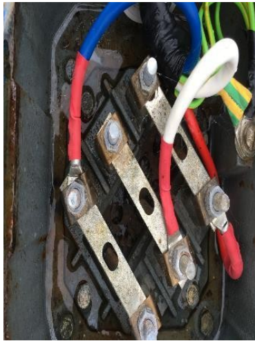
High Resistance due to corrosion
