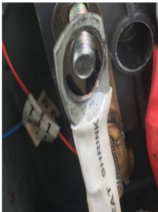
Lug too big poor current path, Heat Shrink Sandwich
