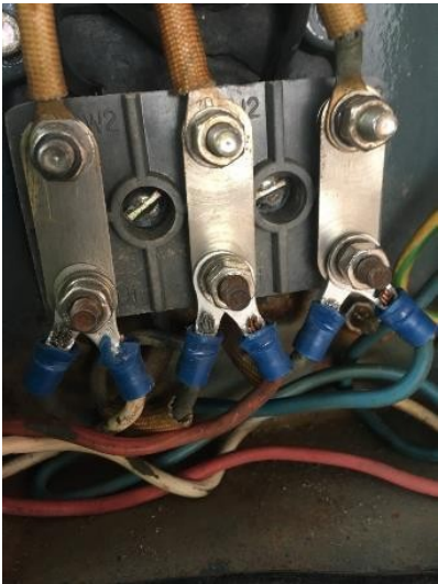
Relugged & Terminated, Denso tape added to terminal box
