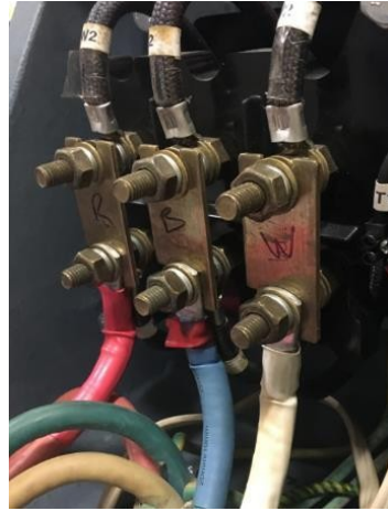
Blue Phase Loose top & bottom. Poor Assembly
