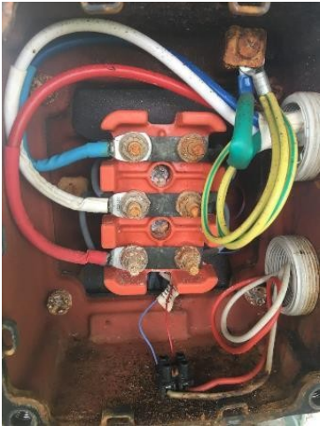
Corrosion, Poor Earth Termination
