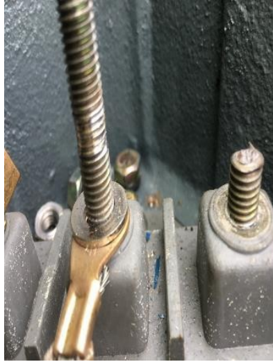
Stripped & Broken studs from poor torque
