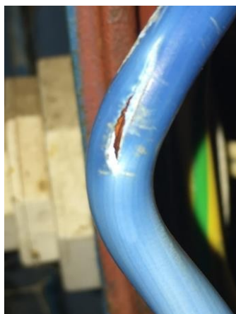
Supply cable damage, bare conductor
