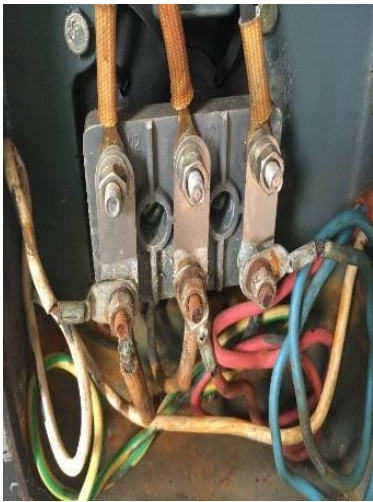
Corrosion High Resistive termination
